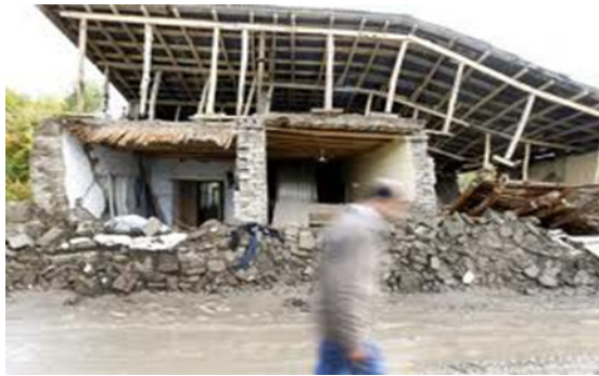
Alakoy Village, Turkey after 7.2 magnitude earthquake June 18, 2010 Photo: upi.com news service
