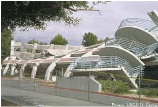
Parking structure - Northridge, CA January 1994 Photo from U.S. Geological Survey
